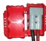
Forklift Battery Connectors
